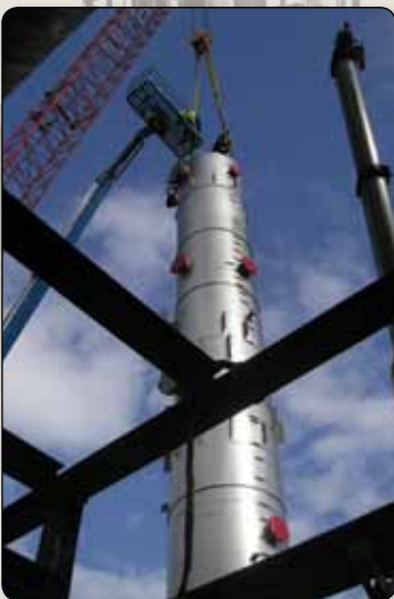
Photo sequence: A distillation tower is lifted into place at the Petro Star refinery in Valdez.
